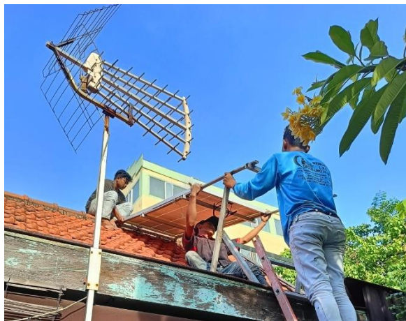
Gambar 5. Instalasi Panel Surya
