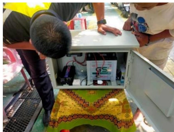
Gambar 4. Box Panel PLTS
